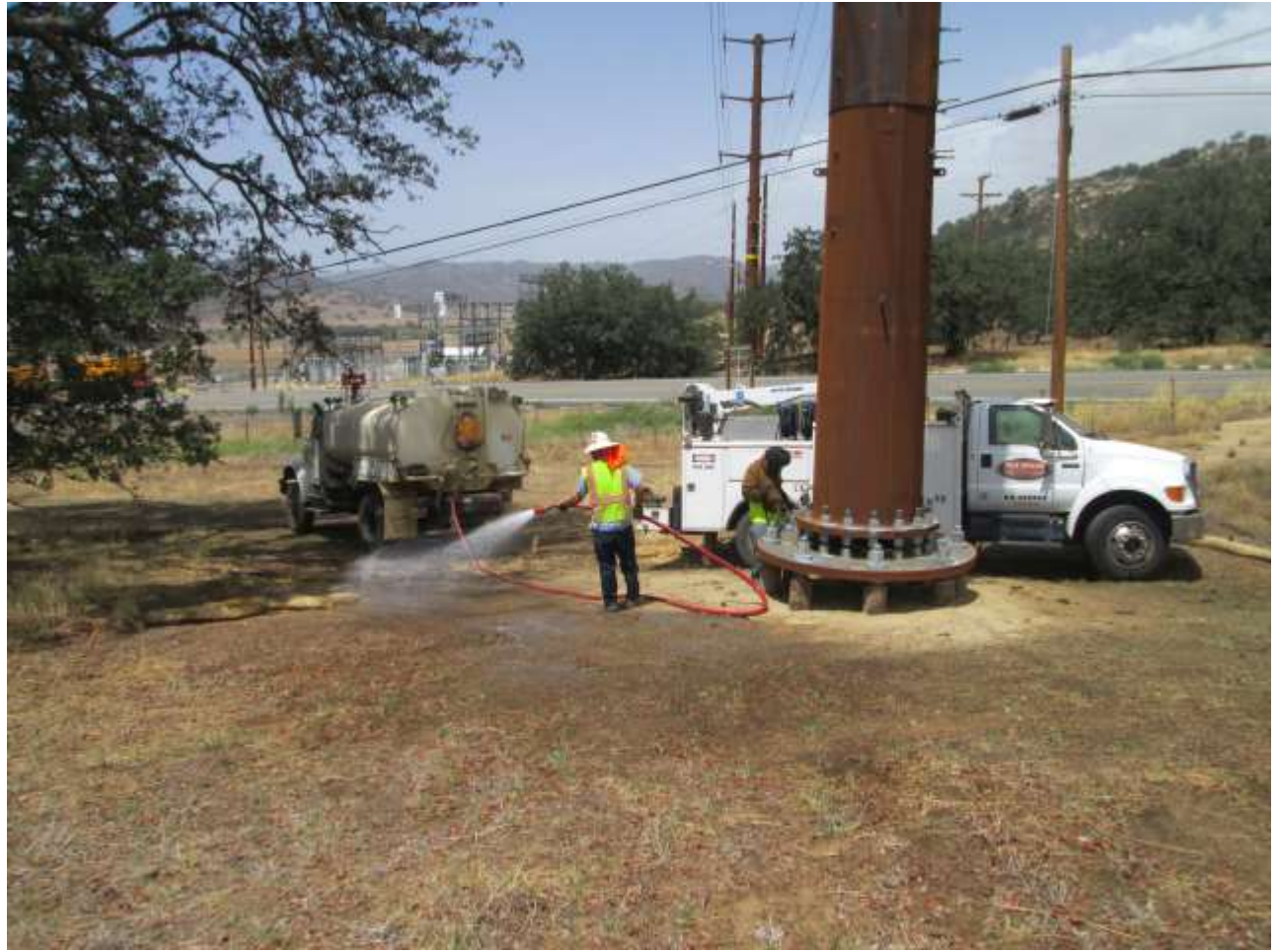
Photo 2: During micro pile foundation nut welding at Location 161, crews were observed watering the adjacent area in accordance with the Project Fire Plan (APM-HAZ-2).
