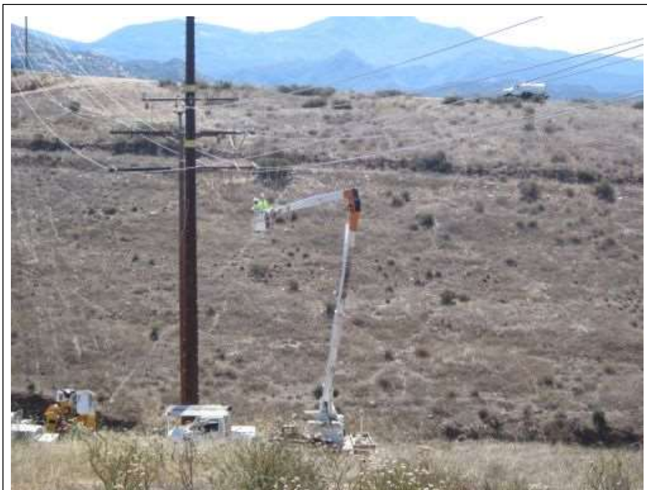
Photo 6: During wire pulling preparation activities (above, Location 28), fire patrols and water tenders (above) were observed monitoring areas along the right- of- way in accordance with the Project Fire Plan (APM-HAZ-2).
