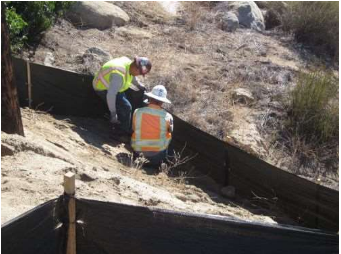
Photo 1: Crews were observed monitoring and repairing SWPPP BMPs throughout the right- of- way. Repairs to silt fencing were observed at Location 35.
