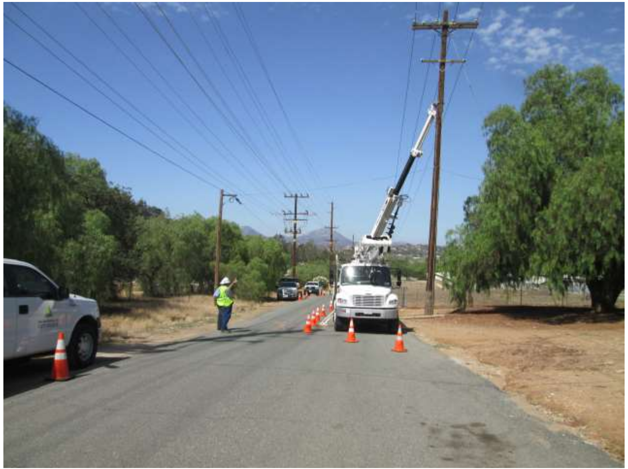
Photo 4: Crews were observed staging water tenders adjacent to activities associated with the removal of the 12kV line along Creelman Lane in accordance with fire safety practices (Project Fire Plan/APM- HAZ-2) and using traffic control measures in accordance with APM-TRA-1.
