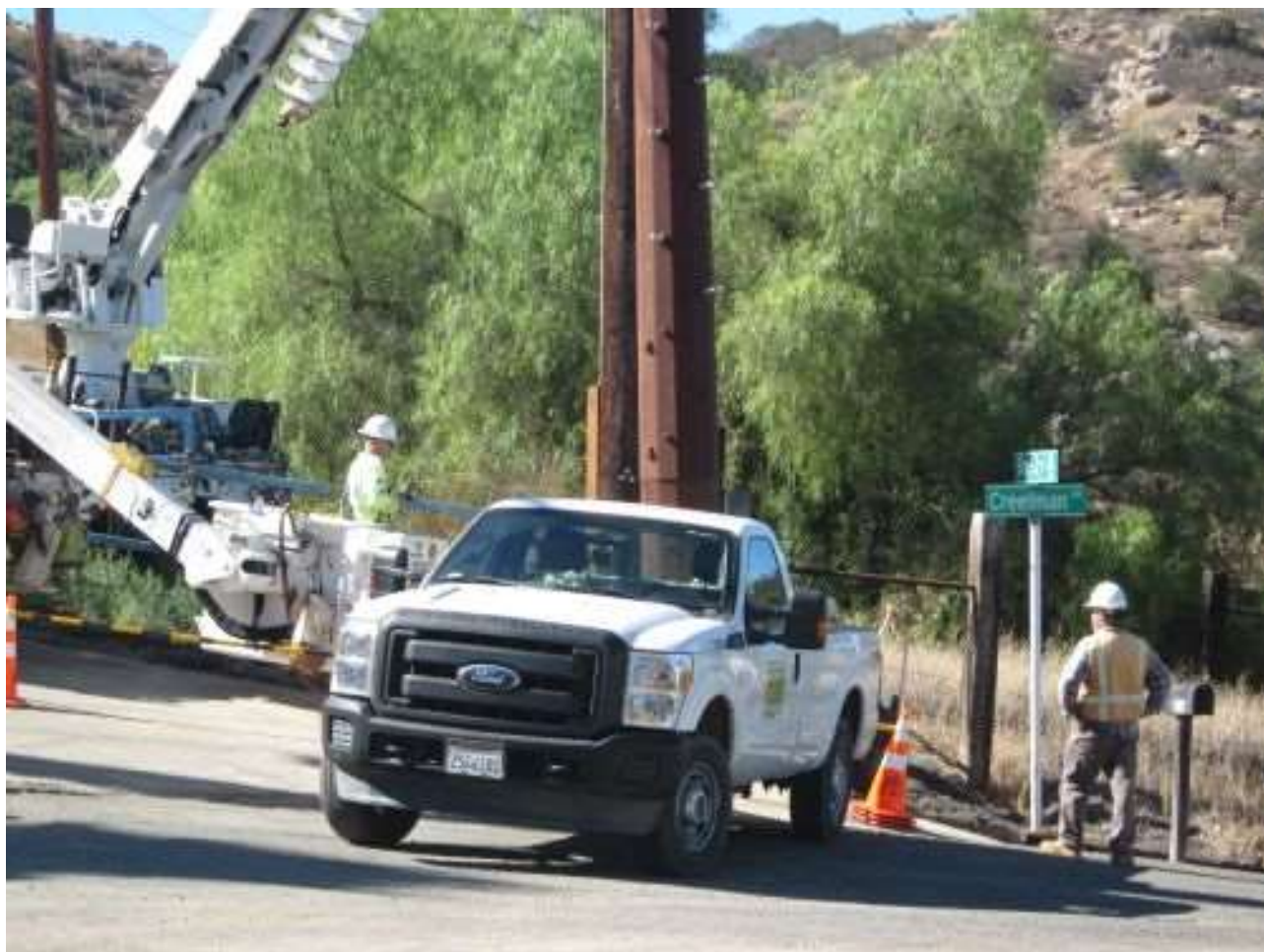
Photo 5: During wire transfer activities along Creelman Lane, biologists were observed monitoring activity in accordance with MM-BIO-2 and ensuring that nesting bird surveys had been completed prior to work occurring at the site (MM-BIO-4).
