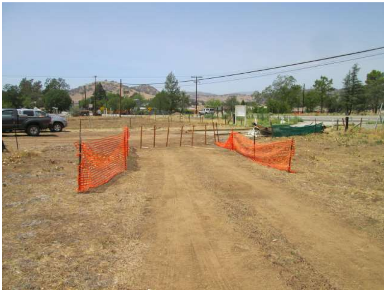
Photo 3: Temporary orange fencing used to delineate avoidance areas for sensitive plants (San Diego Gumplant) was observed intact and plants were avoided by construction crews in accordance with MM-BIO-1.
