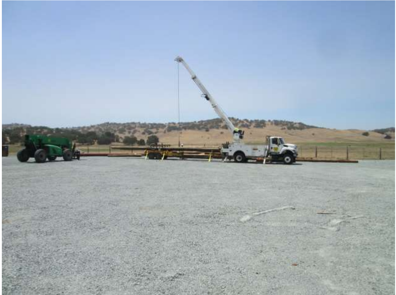
Photo 7: At the Santa Ysabel Staging Yard, crews were observed loading decommissioned wooden poles for hauling off site.
